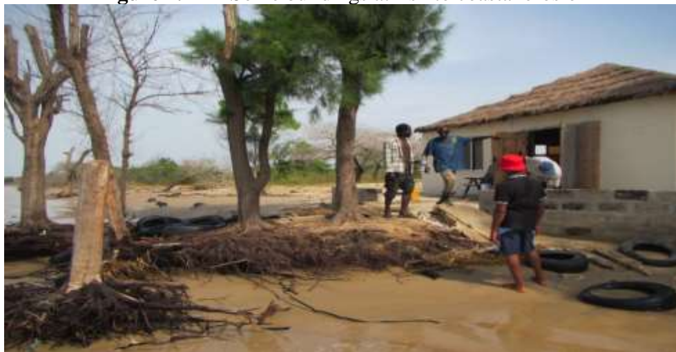
Figure 4.4 Some buildings at risk to coastal erosion
