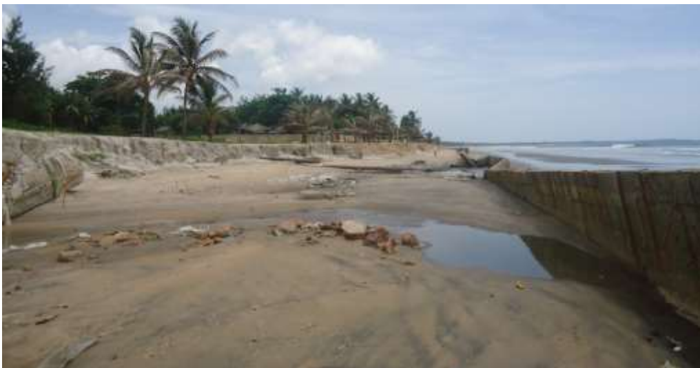
Figure 4. 10 Seawall Over-topped by SLR and coastal erosion
