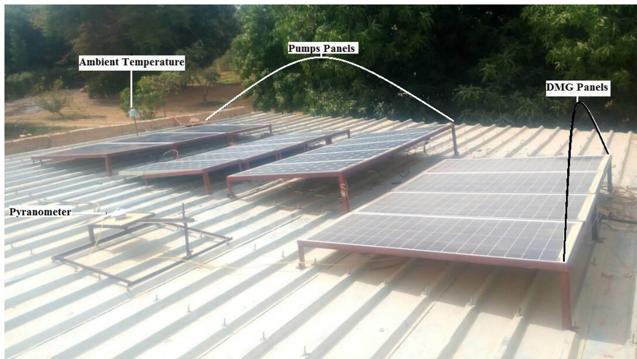
Figure 3-4: Photography of the pump and DMG panels, pyranometer, and ambient temperature shelter.
