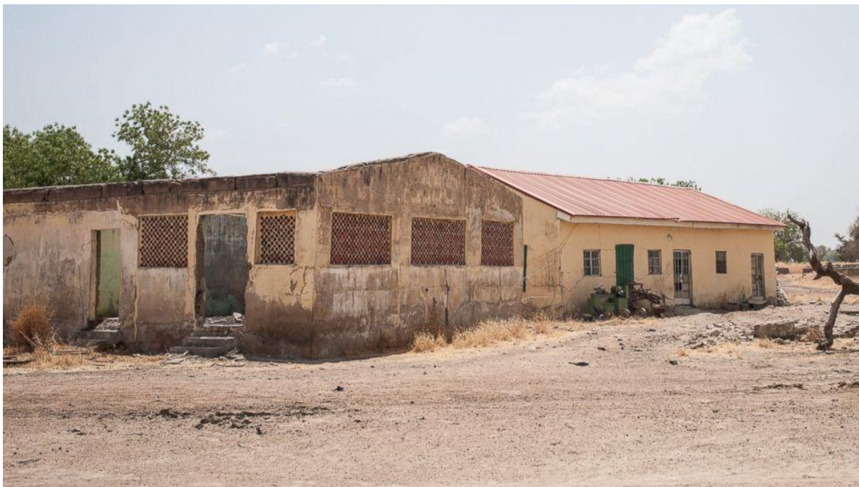
Plate II: A dilapidating building in Chibok Local Government Area, Borno State
